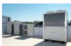
2012 New GHP units. Panasonic's gas-driven VRF Systems are ideal for projects where power restrictions apply.
