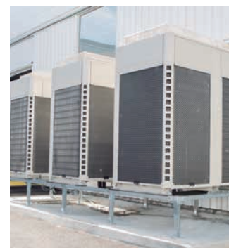
Skobe Volvo with high energy savings of up to 65%. Katrineholm, Sweden. PACi and VRF
