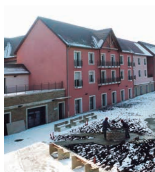
Montcenis Nursing Home. Over 6.100 m 2 and 85 rooms. Saône et Loire, France. ECO-G
