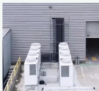
STEMCELL Technologies, a global biotechnology company, installed CO 2 condensing units - CR Series for cold rooms in the warehouse. France. Refrigeration
