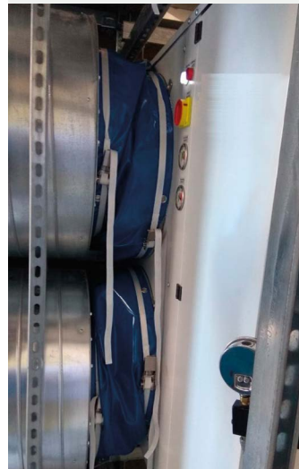
High pressure fan.
