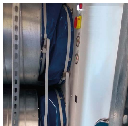
High pressure fan.
